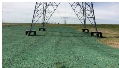
Figure 2. High disturbance site where soil is stripped, piled, and replaced up to 8 months later and reseeded.
